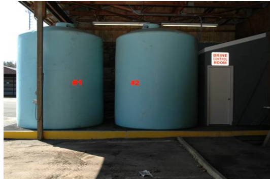
Figure 28. Proper Brine Storage
